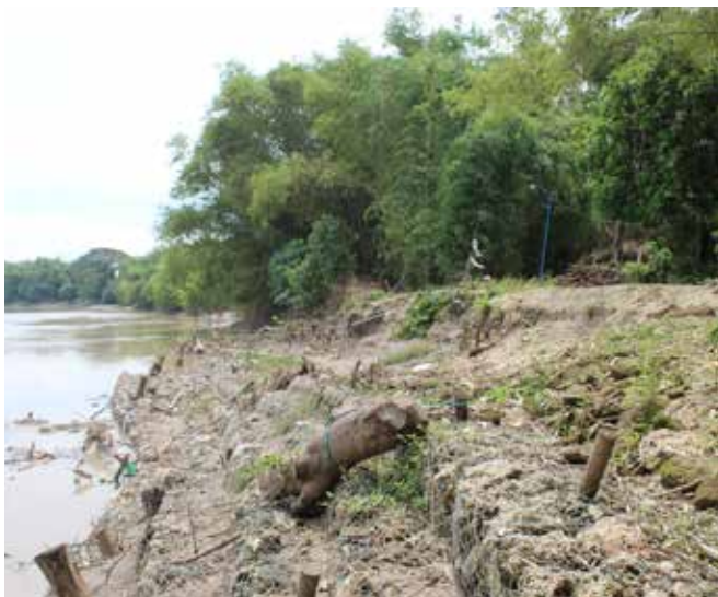
The land in Mlaten Hamlet which has been supported by gabions is still being eroded. In the distance, bamboo groves appear to be more able to protect the land from erosion.
