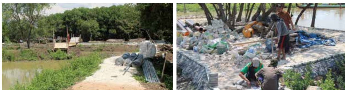
A number of workers are busy working to build the conservation-based mangrove tourism area in Pangkahkulon Village.
